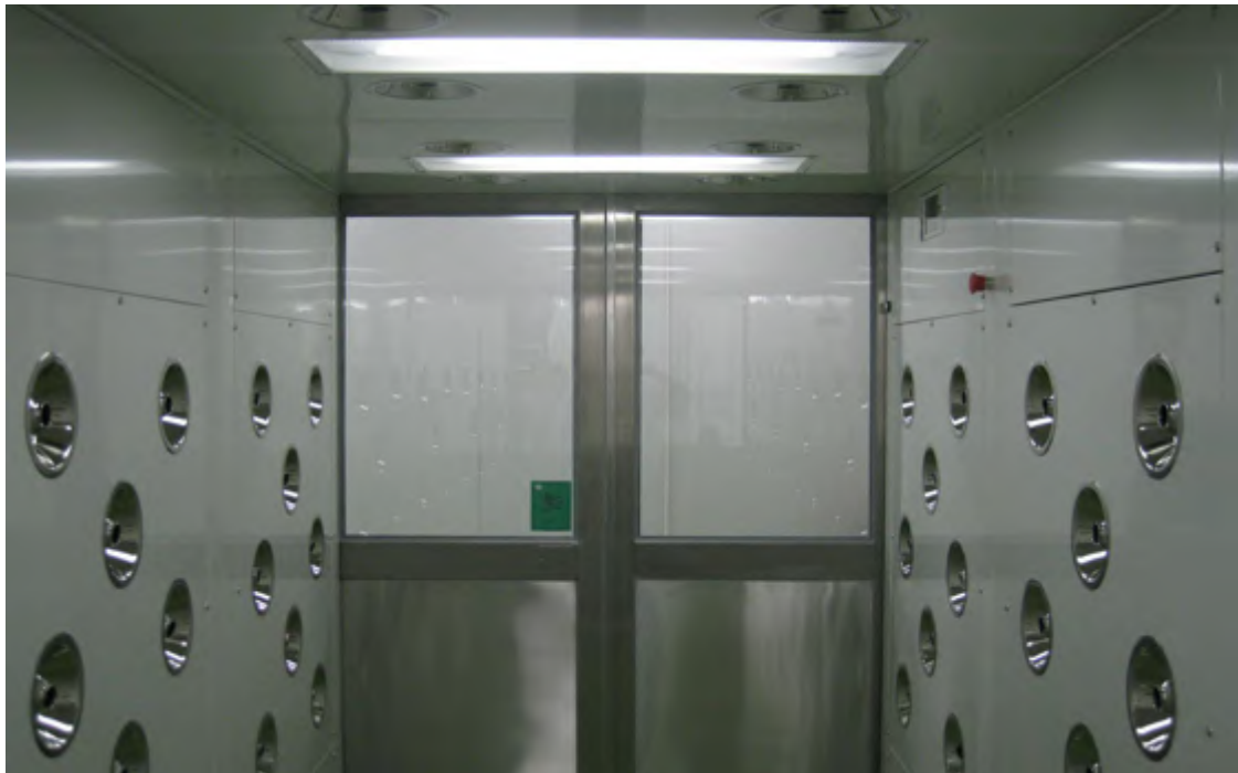
Air shower room
